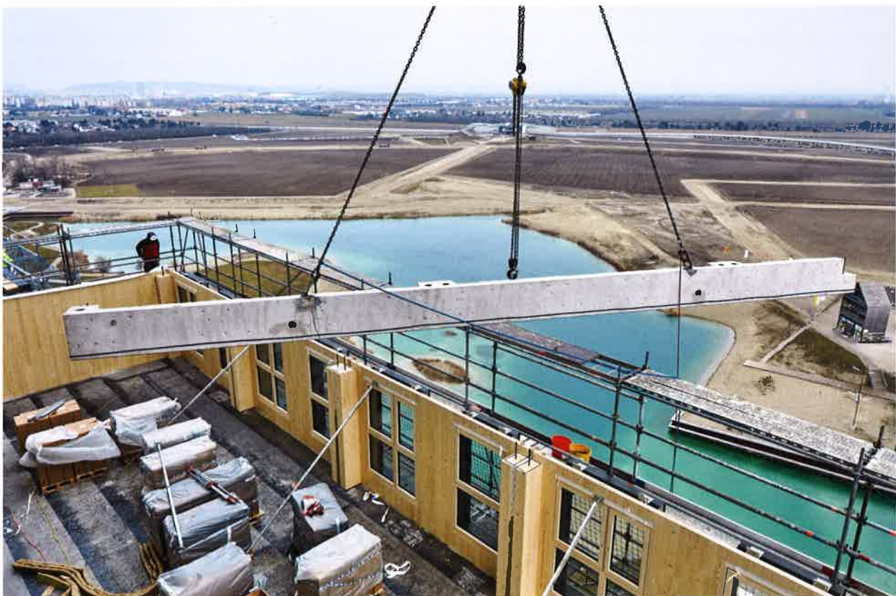
Concrete ring beam placed on top of the prefabricated column and wall panels below
