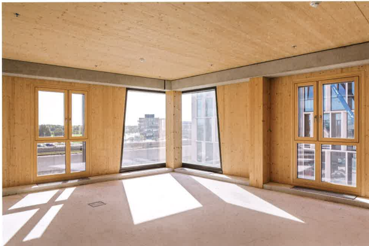
Interior with exposed CLT floor as ceiling finish, concrete ring beam and spruce wall panels
